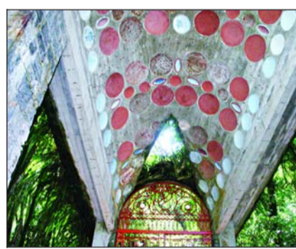
Arches and gateways that lead nowhere are among the many mysterious structures left by James in Las Pozas.
